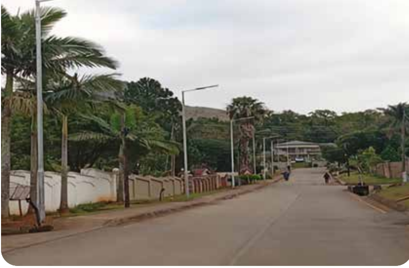
Figure 1: Installed solar streetlights at Hospital Street.
