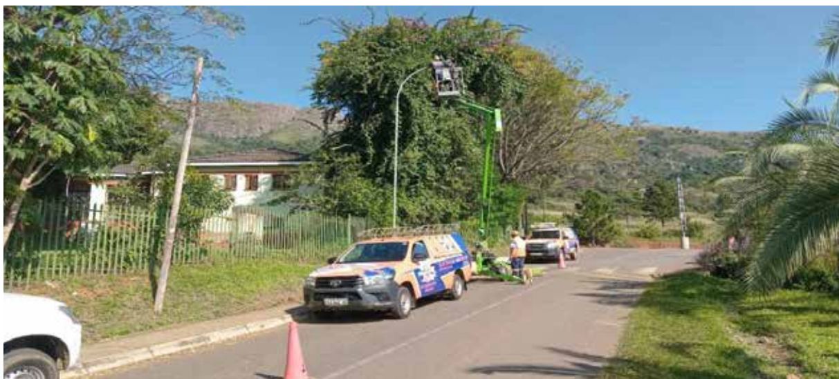
Figure 3: Conversion of HPS to LED lights along Mpumalanga Road.
